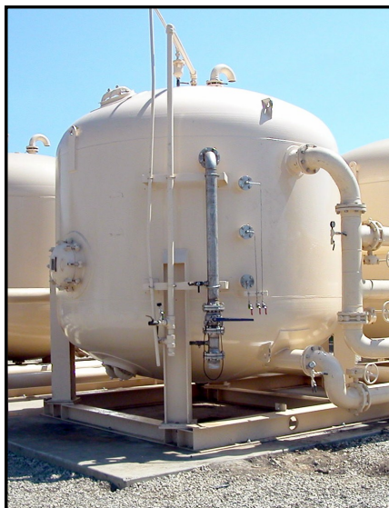
Figure 2: GAC Water Treatment System
