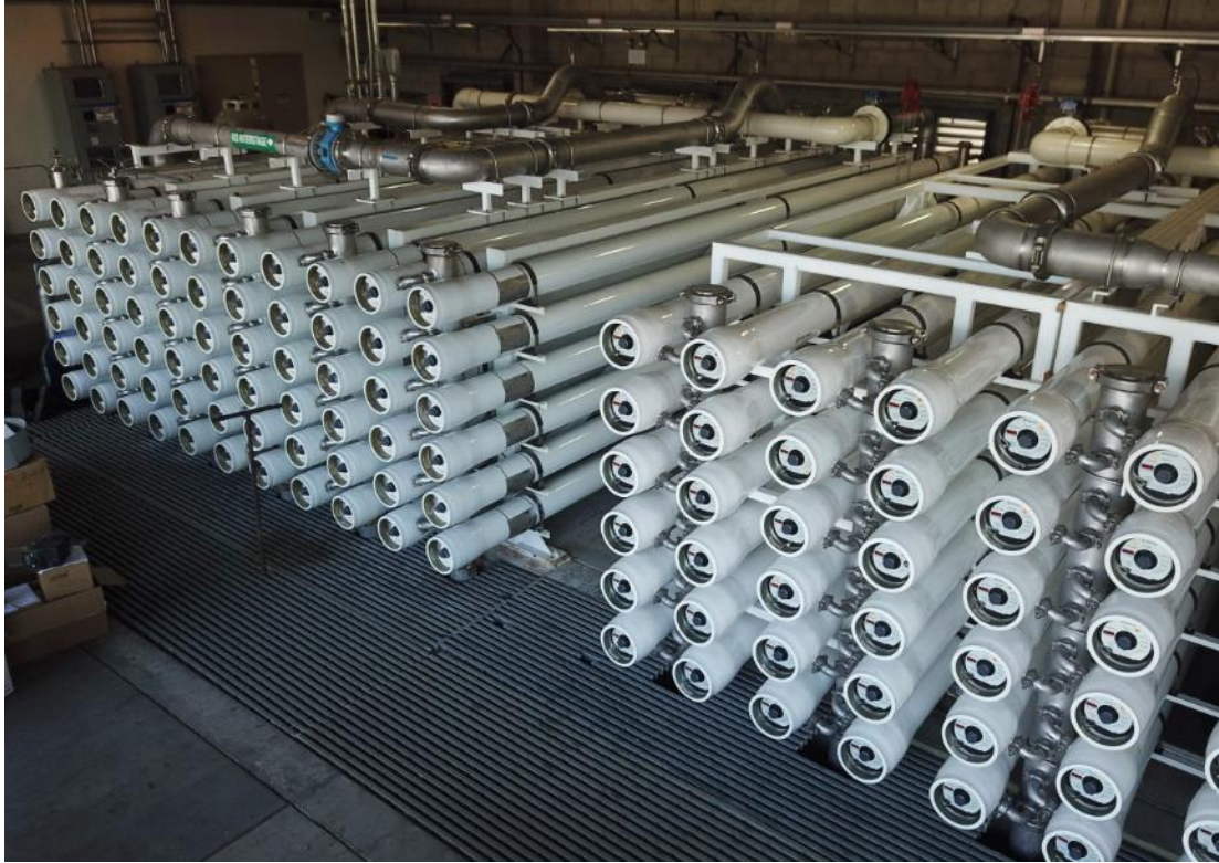
Figure 9-3: RWGD Reverse Osmosis Equipment Indoors
