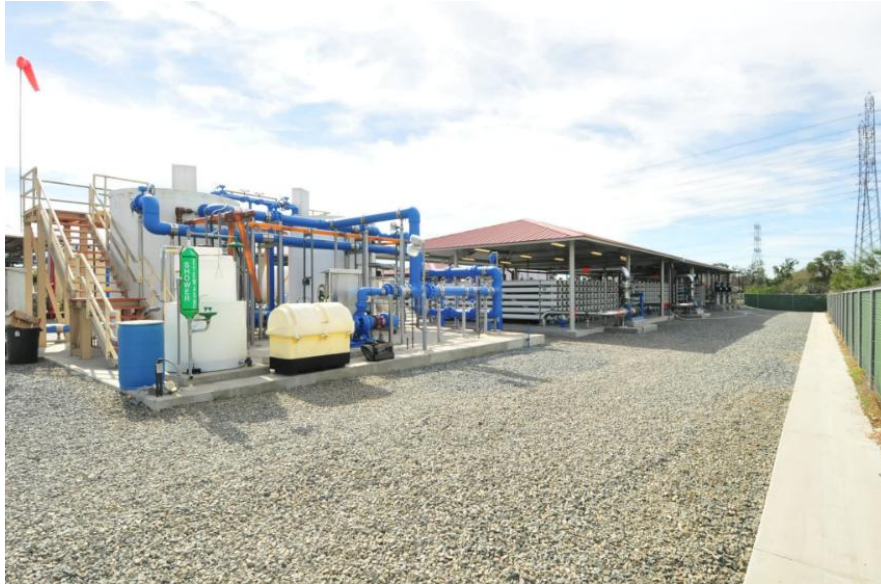
Figure 9-1: LVL Gravel Surrounding On-Site Equipment
