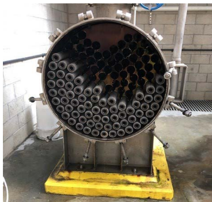
Figure 5. Fouled Cartridge Filters prior to Replacement on September 16, 2020
