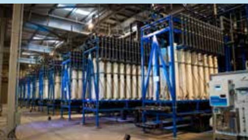
ARC's filtration process will produce approximately 10,000 acre feet (3.25 billion gallons) of recycled water annually to near-distilled levels.
