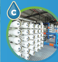
Leo J. Vander Lans Advanced Water Treatment Facility
