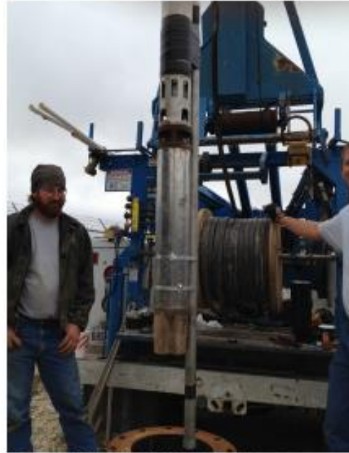
Figure 3: Stainless Steel Pipe attached to pump
