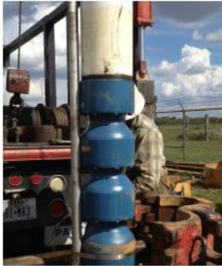
Figure 2: Riser banded to pump bowls
