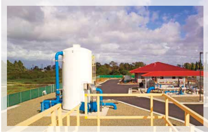
Leo J. Vander Lans Water Treatment Facility in Long Beach, California
