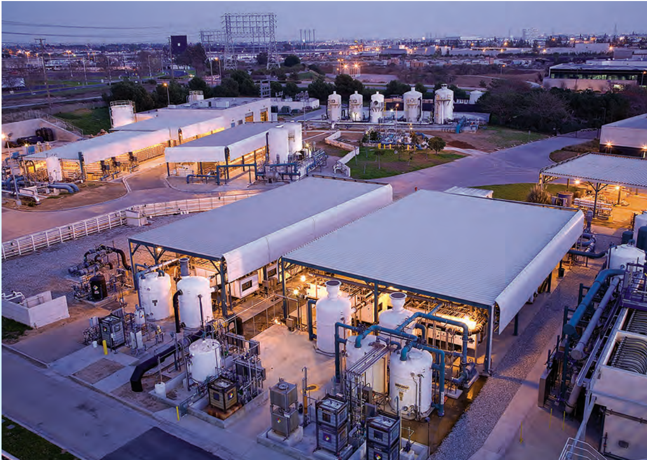
West Basin Municipal Water District's Ed C. Little Water Recycling Facility in the City of El Segundo Image courtesy of West Basin Municipal Water District
