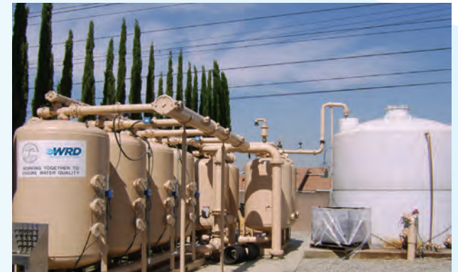
Wellhead treatment system in the City of Paramount
