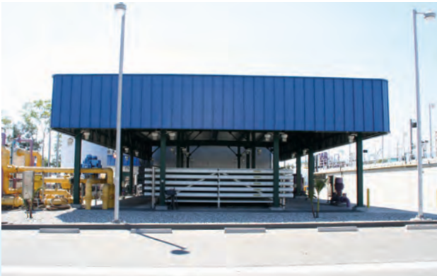
Los Angeles Terminal Island Advanced Water Purification Facility Image courtesy of City of Los Angeles
