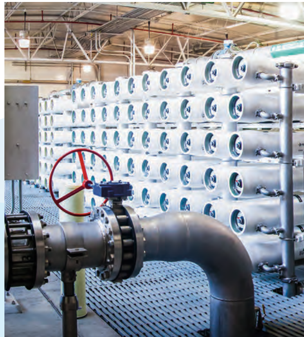
Energy recovery devices are installed at pumps at the Goldsworthy Desalter in Torrance.
