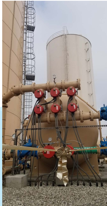
Pictured is the water treatment system installed at a water production well at Maywood Mutual Water Company No. 2.
