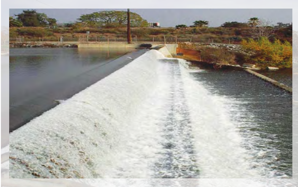
Rubber Dam at the San Gabriel Spreading Grounds
