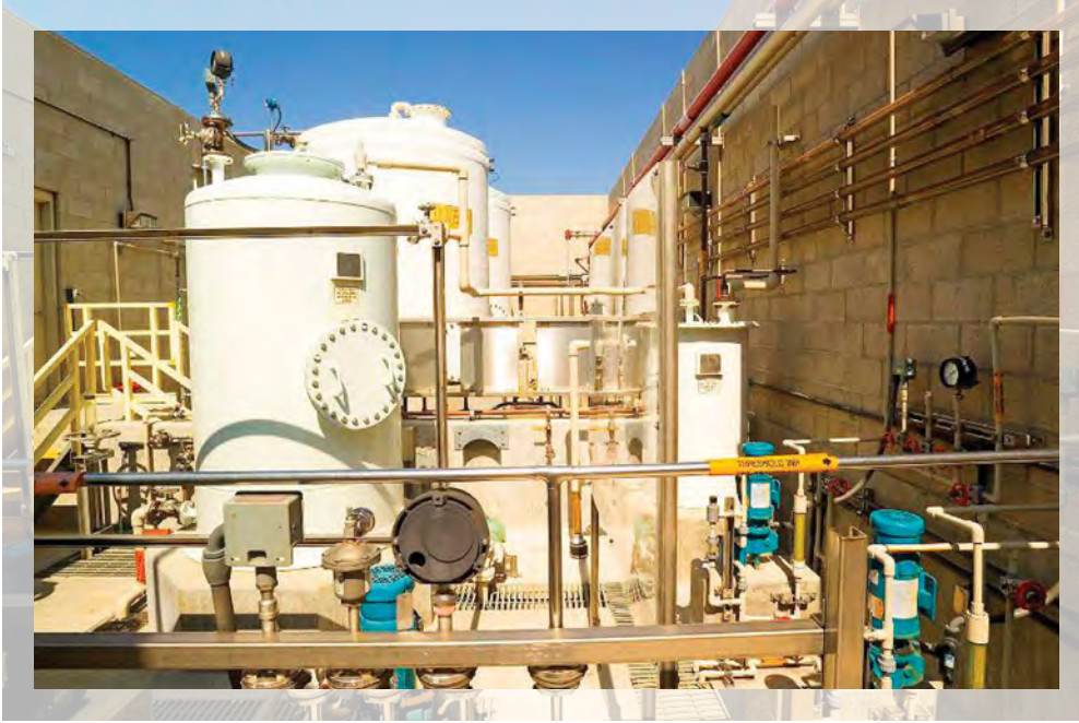
Robert W. Goldsworthy Desalter in Torrance, California
