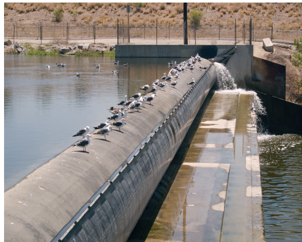
Rubber dams on the San Gabriel River can be inflated to retain water for infiltration into the substrate below the river's channel or can be deflated to facilitate flood control measures, 2007. Image from the WRD archives.
