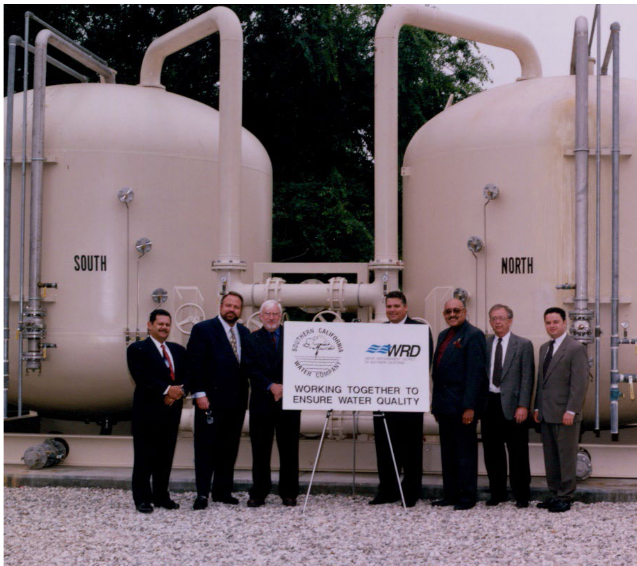
Groundwater treatment equipment at one of WRD's Safe Drinking Water Program projects. From left: Three officials from the Golden State Water Company, WRD general manager Robb Whitaker and directors Willard H. Murray, Jr., Robert W. Goldsworthy and Albert Robles. Image from the WRD archives.
