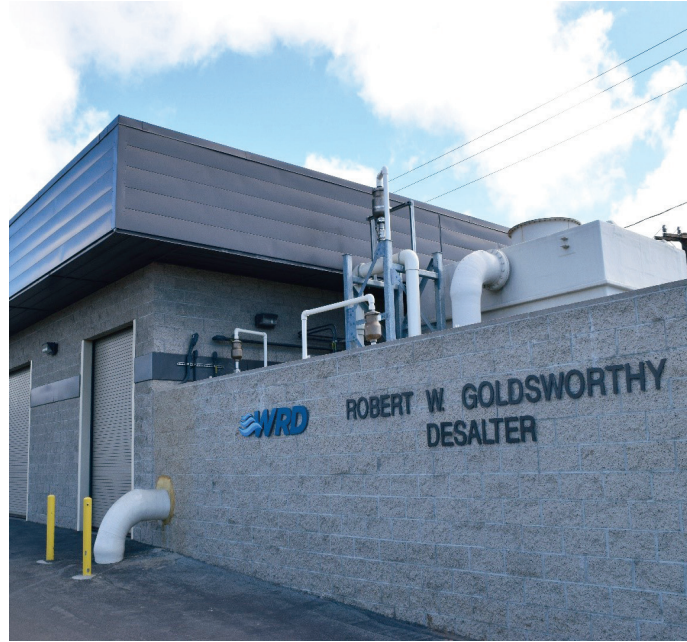
WRD's groundwater desalter in the city of Torrance, 2018. Image from the WRD archives.
