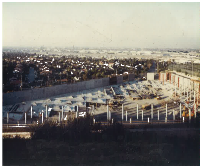
Haggott Reservoir nearing completion, ca. 1987. Image courtesy of the city of Torrance.
