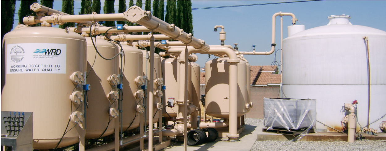
Wellhead treatment equipment for the Southern California Water Company's (now Golden State Water Company) Century Well in Paramount, CA, 2006. Groundwater is pumped to the surface and is treated for iron, manganese and arsenic through the use of chlorination, oxidation, adsorption and filtration. Image from the WRD archives.
