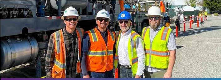
Director Katherman at a site visit during the installation of a new pilot testing well in the City of Torrance.
